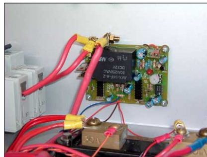
The circuit board in Ross's system. We recommend mounting it inside an insulated enclosure if you can.
