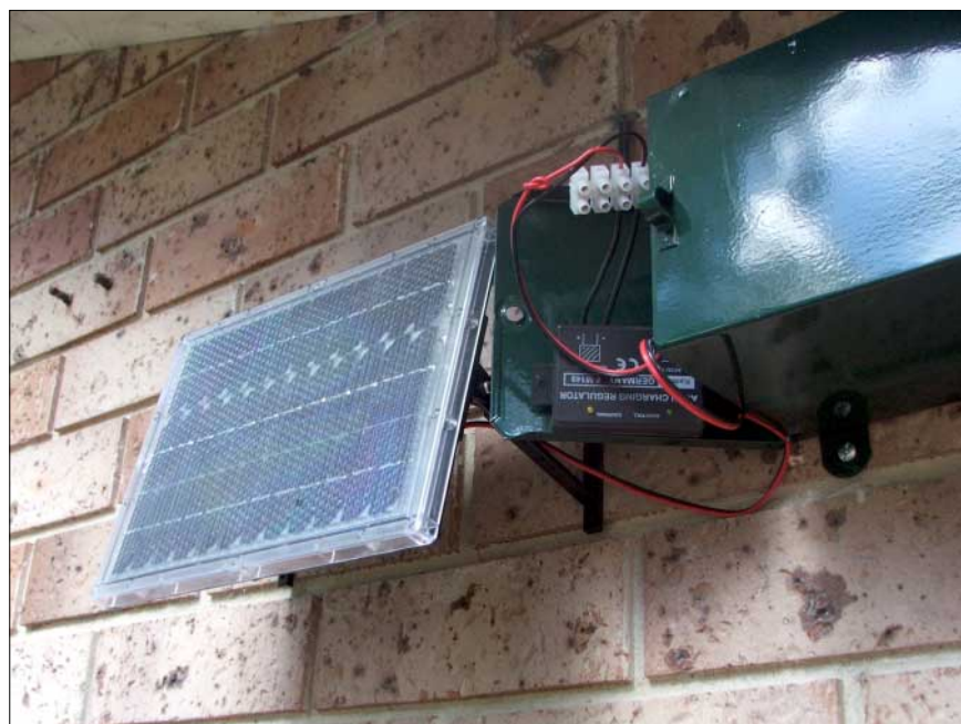
The solar panel, mounted next to the box holding the battery and charge regulator.
