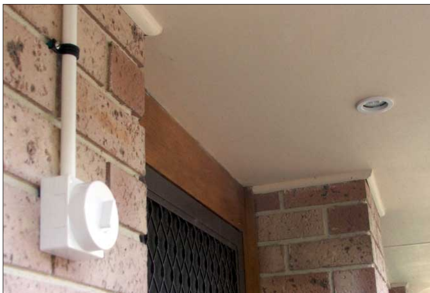
The switch (bottom left) used to turn on the LED porch light (top right)
