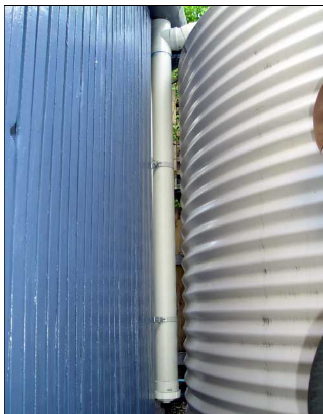
Top: Designated hose for recycled water. Bottom: The rain diverter captures the first few litres of rain that may contain pollutants.
