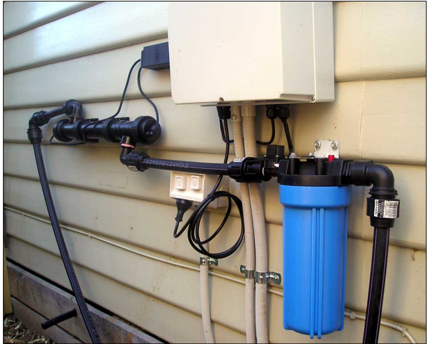
The water passes through a particle filter and then an ultraviolet light which disinfects the water.
