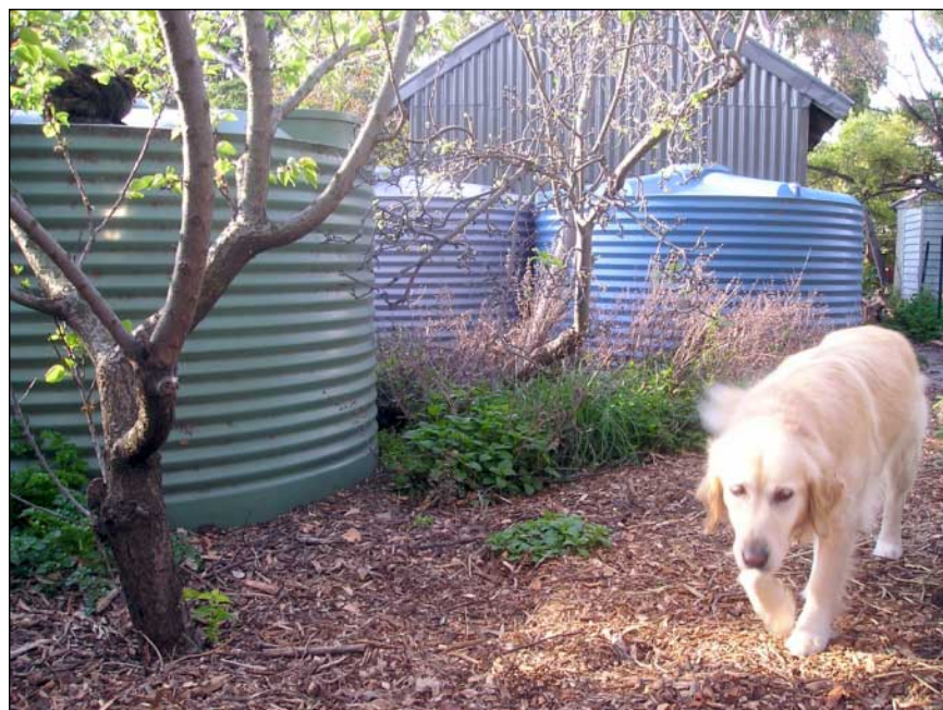
Four rainwater tanks store up to 20,000 litres of water and supply about 60% of the McQuire's water needs.
