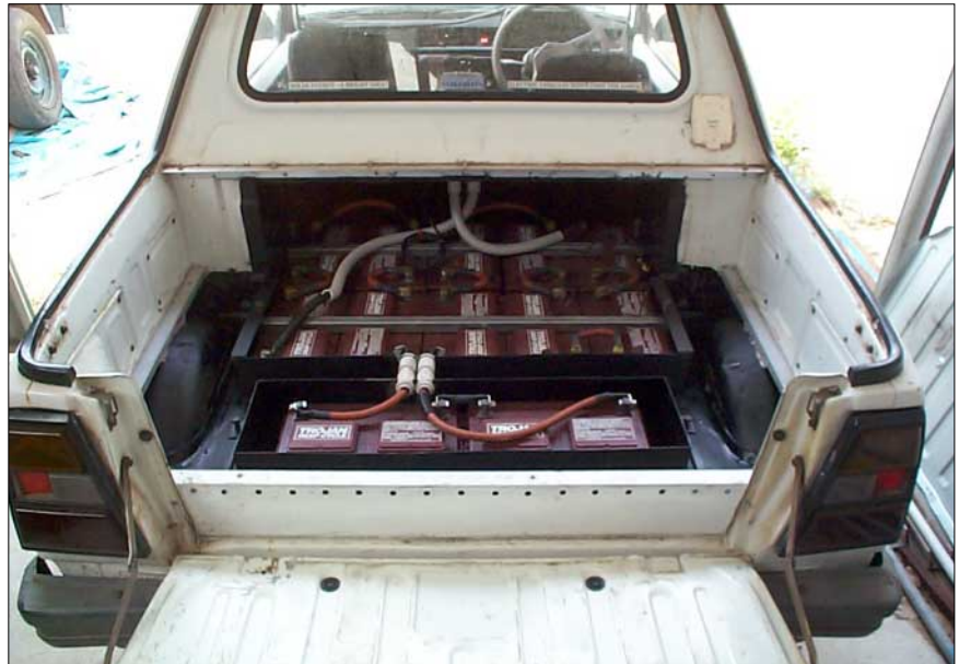
The batteries are mounted under the tray, so the cargo area is still fully useable.
