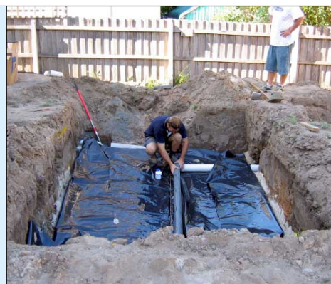
3. Paul Talbot lays the collection pipe to the base of the sand filter.
