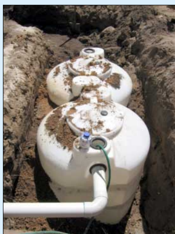
5. Settling tanks gravity feed the greywater into the sand filter.
