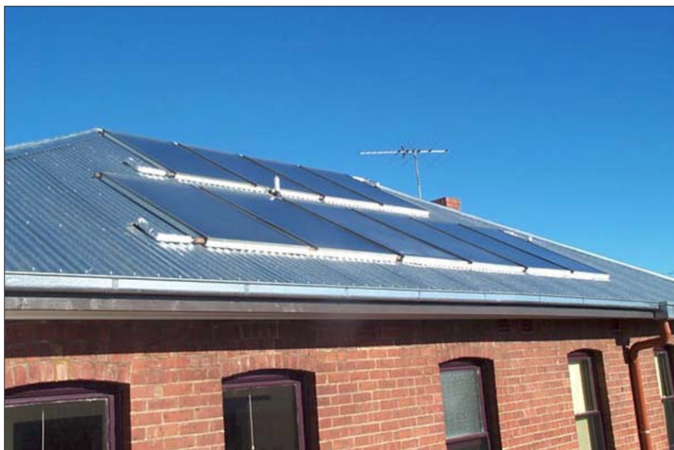
The hot water solar collectors on the roof of the Beach House.
