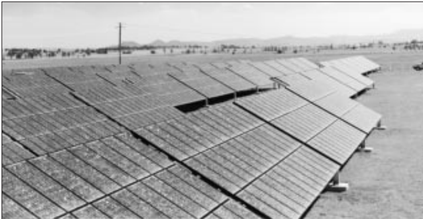
Stage one of the Singleton solar farm: 200 kW of Solarex panels.
