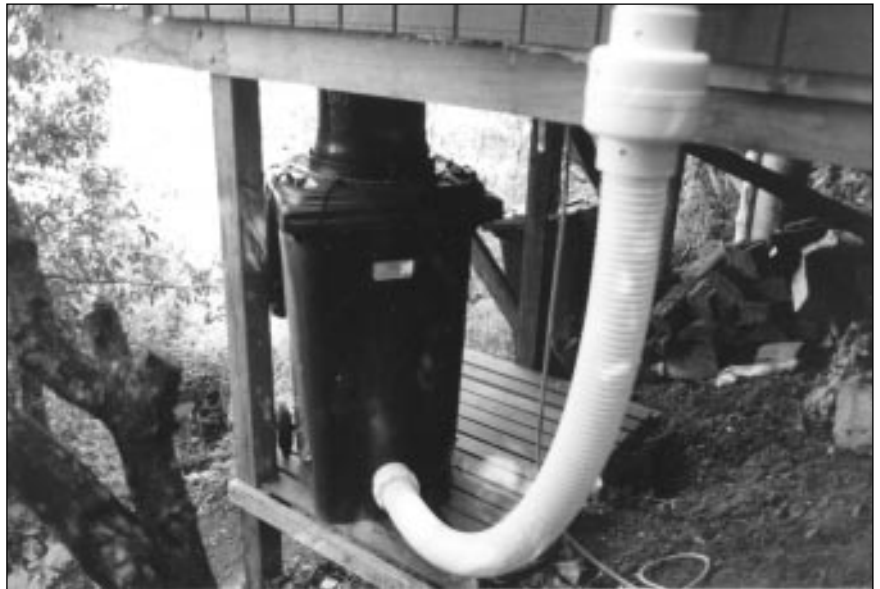
Designing your house to suit can make fitting a composting toilet much simpler. Excavating after the house is built can be a costly exercise.
