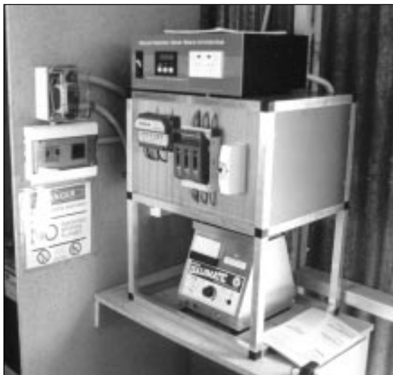
The control centre of a combination ELV and LV RAPS system. The 240 volt AC wiring is on the wall at left, while the ELV DC wiring is completely separate in the enclosure.
