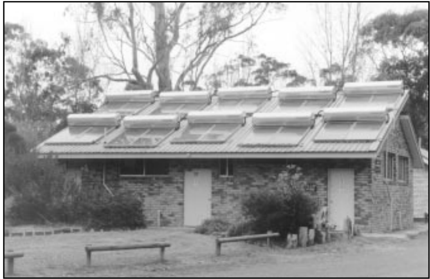
That's a lot of hot water! These solar water heaters provide the hot water for half of this shower block in the Grampians.
