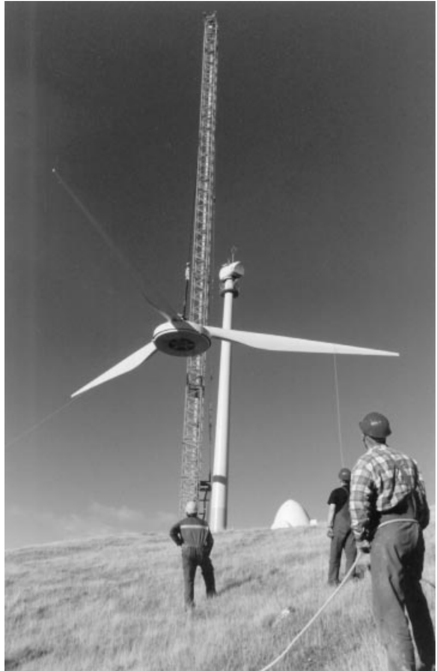
Hoisting a blade assembly on to its tower at the Haunui wind farm.
