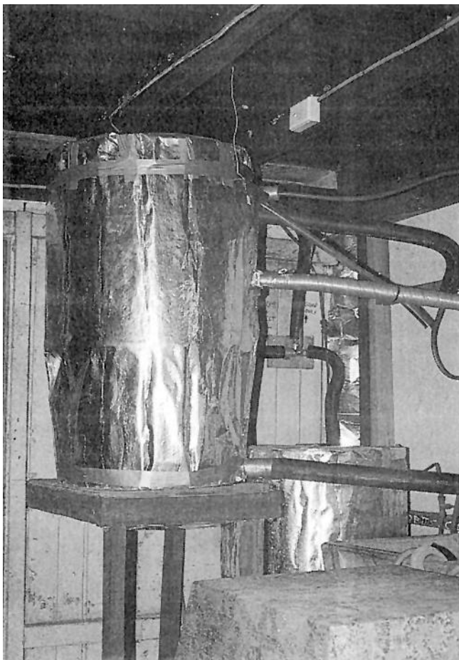
Solar tank (higher) and electric tank located under the house.
