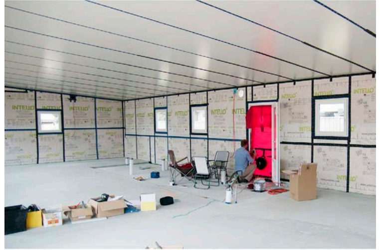
↑ Blower door testing ascertains envelope airtightness by sucking internal air out through the door and testing for any air infiltration into the building through gaps.
