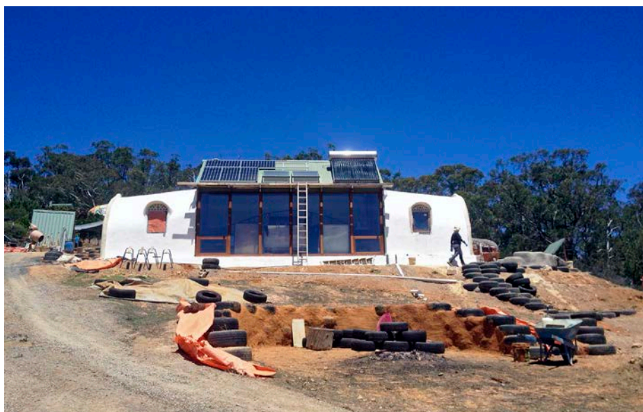
↑ Martin's almost-completed earthship in Ironbank, in the Adelaide Hills, South Australia. The design is based on the Simple Survival Model, adapted for use in Adelaide's warmer climate. The north-facing greenhouse sits in front of the main room which serves as bedroom, living area and kitchenette. An airlock entry room is at the east end of the greenhouse, and a bathroom at the west.
