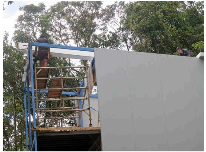
↑ The SIPs were light enough to be lifted by two people and set in place by four.
