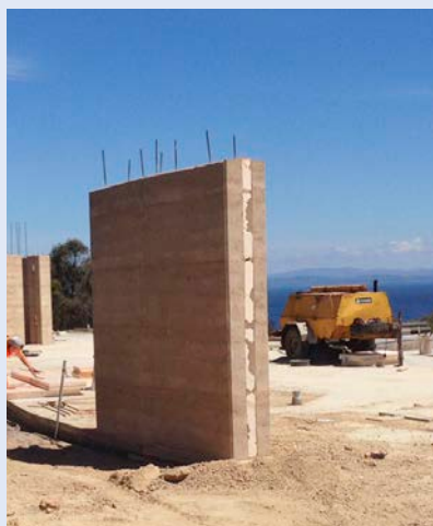
↑ Insulated rammed earth wall section, with 175mm rammed earth each side of a 100mm styrofoam core.
