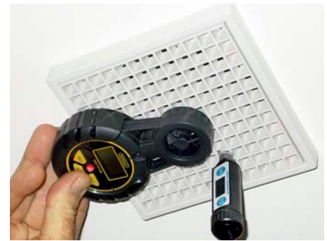
↑ Measuring the airflow and air temperature at one of the five eggcrate ceiling vents. The little digital anemometer is typical of those readily available for under $100.
