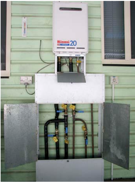
↑ Three options of hot water plumbing: gas-boosted solar, full gas and solar only.
