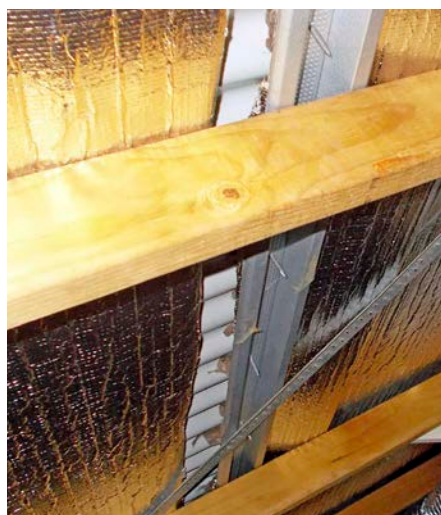
↑ A 10 cm strip of sisalation is cut out along the roofline, 800 mm below the roof peak. Note the Insulwool at the top edge of the cut.
