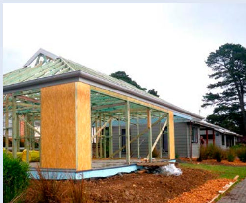
↑ Granny flat under construction, showing timber framing, roof trusses and the concrete slab with insulated edges, with the main house and carport in the background.
