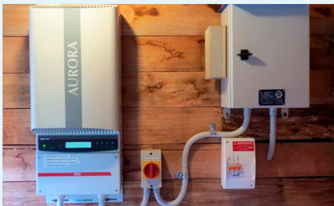
↑ The grid-interactive inverter is on the left. On the right is the micro-hydro turbine controller.
