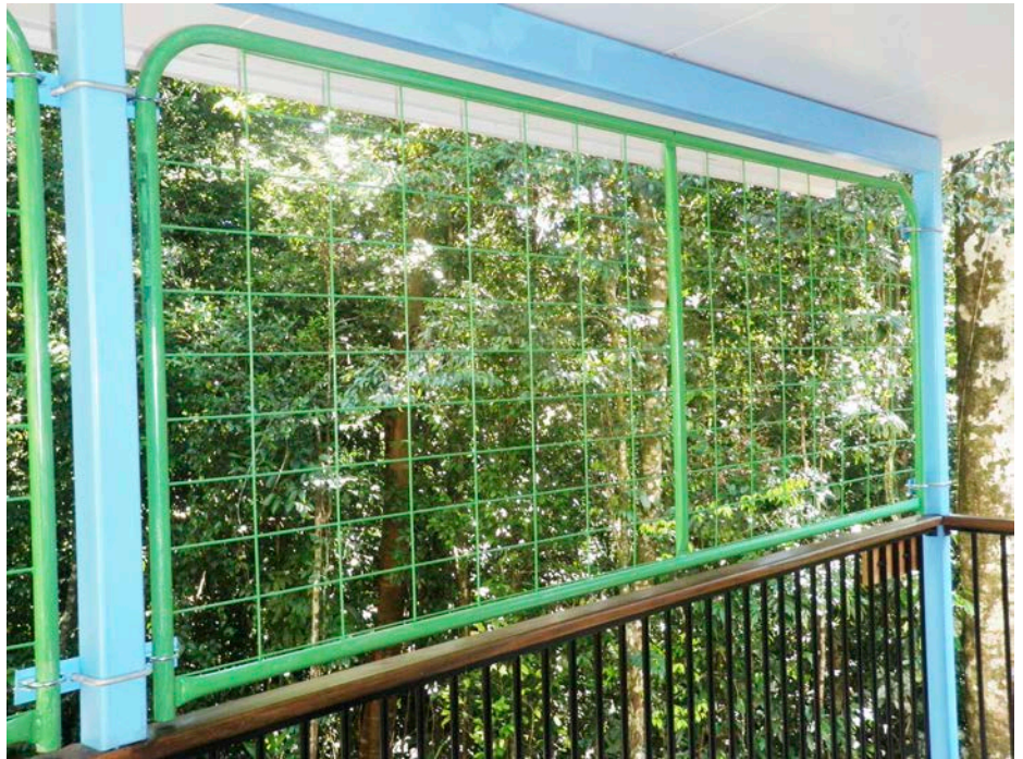
↑ For seasonal cyclone protection, they attach standard farm gates on top of the balcony railing. They are installed a few hours before a cyclone is due and taken down shortly after.
