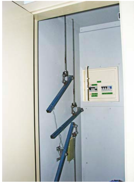
↑ Levers are used to control ventilation ducts.
