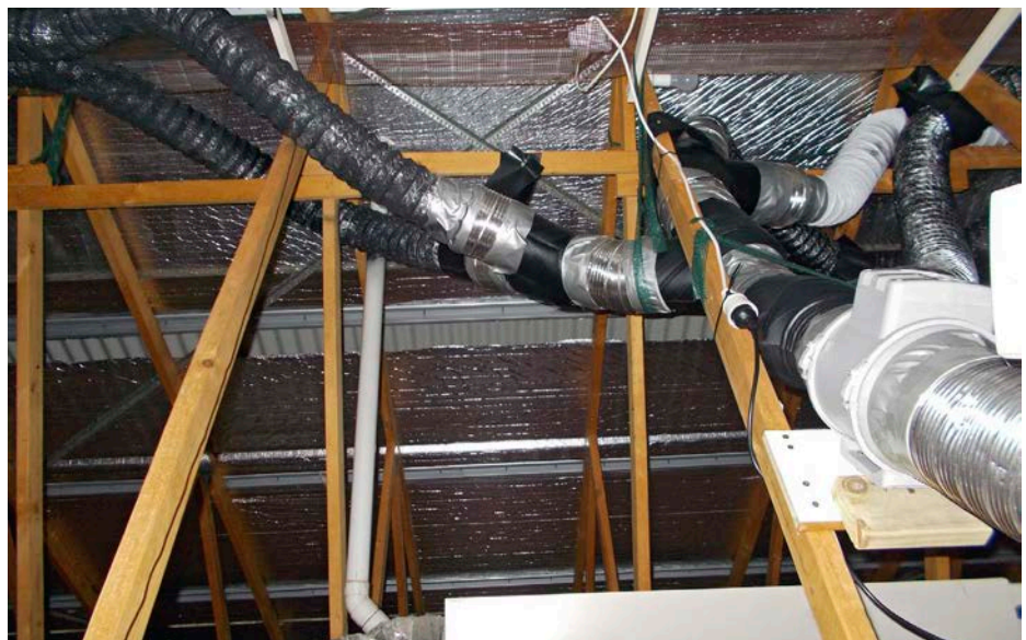
↑ A 150 mm inline fan (white object in the ducting at right) distributes air to five 12-metre runs of black-painted 125 mm aluminium flexible ducting.
