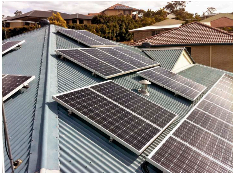
↑ The 12kW array was split into two separate 6kW arrays, each connected to its own inverter.
