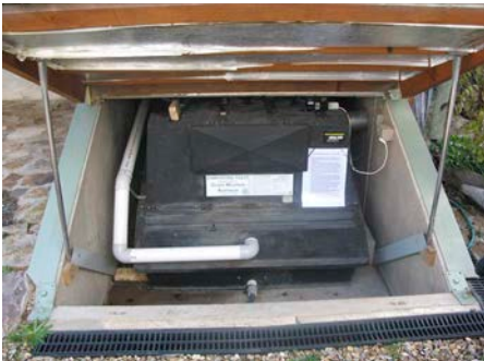
← The compost processor—note the warm air feed (white pipe) from the house to keep the compost pile warm and ensure continued composting, especially during the cold of winter.
