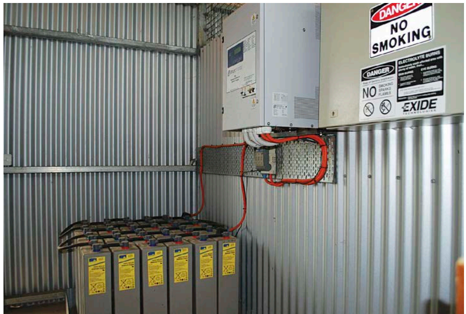
↑ The inverter and battery bank are located in an insulated section of the vehicle shed, to keep the batteries cool and the potentially annoying cricket-like chirruping of the inverter away from the house.
