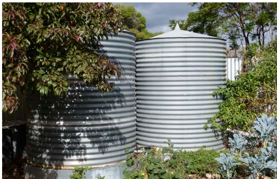
↑ Three secondhand (ex Housing SA) 4500L galvanized iron tanks are linked to provide water for the house and garden. Rainwater for drinking is provided by a separate 1000L tank.
