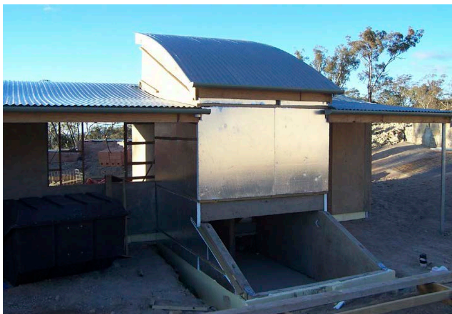
↑ The composting toilet under construction, with insulation around the edge of the service pit.
