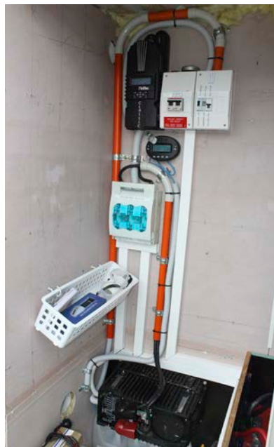
↑ Charge controller, inverter and isolators.
