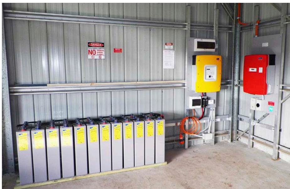
↑ A typical AC coupled off-grid system. The battery bank is on the left, the yellow box is the inverter/charger and the red box is the grid-interactive inverter.
