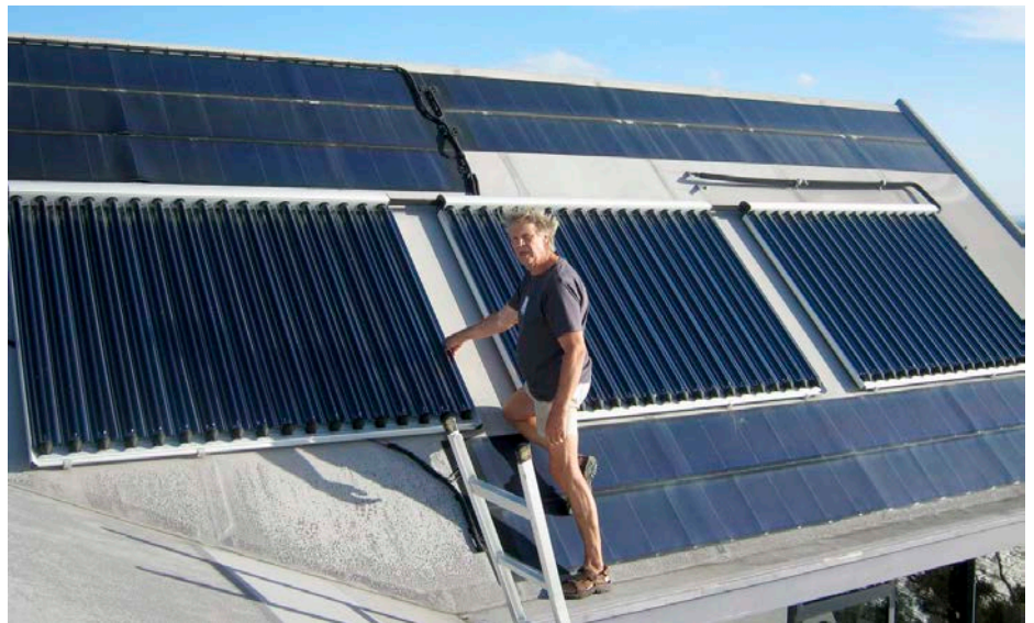
↑ Chris's house, located near Coromandel Town in New Zealand, has 9m 2 of hot water collectors mounted between UniSolar PV panels. These are 'U-tube' type tubes, with the circulating water contained within small copper tubes inside the vacuum tubes.
