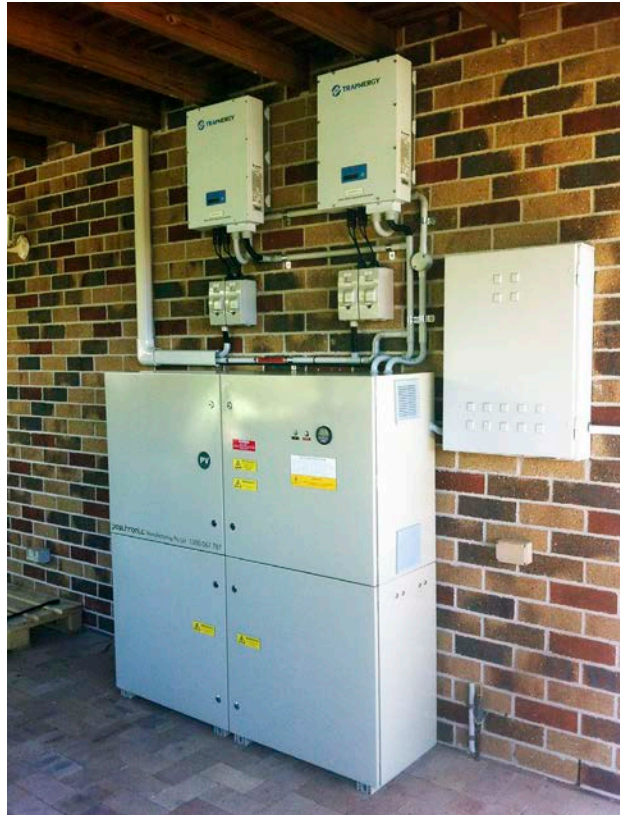
← The complete system. The ESS (energy storage system) makes for a very neat installation, quite small for 29kWh of battery capacity.
