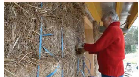
↑ A willing volunteer helps to make the strawbale walls of Dana and John's new house.
