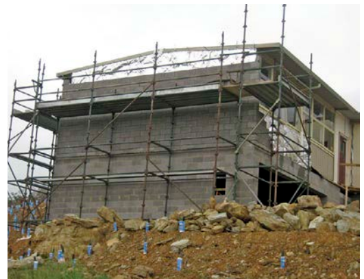
↑ The blockwork going on one of the portables, with foil insulation underneath.
