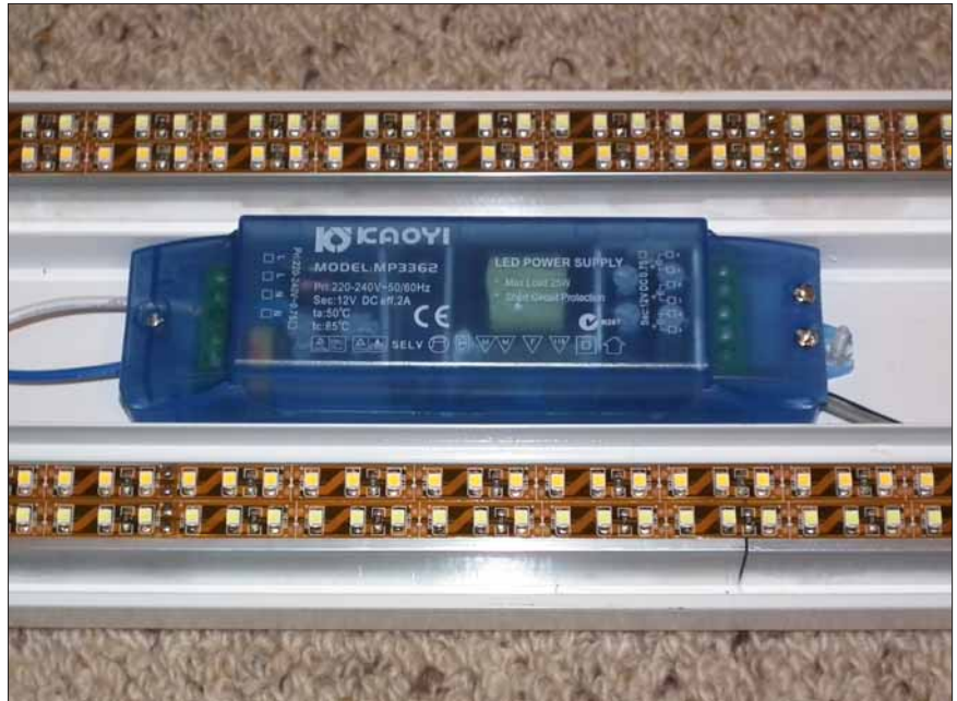
The new power supplies fit neatly where the old ballast used to, almost like they were made for the job! Note how the LED ribbon is mounted on square aluminium tube.
