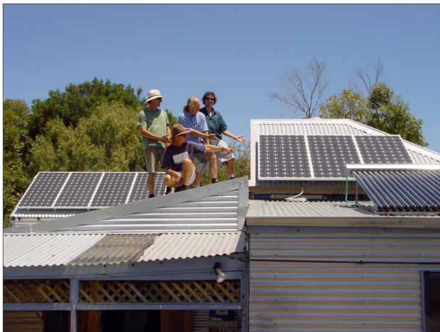
Residents with some of the first photovoltaic systems installed in Hulbert Street.
