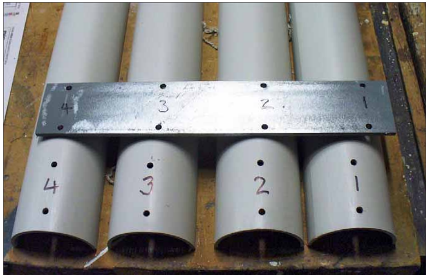
The plates are drilled and then used as a template to drill the pipes.
