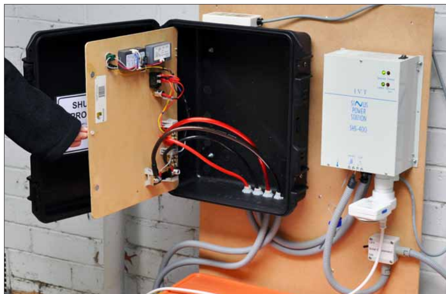
Inside the control box. There's plenty of space for expansion.
