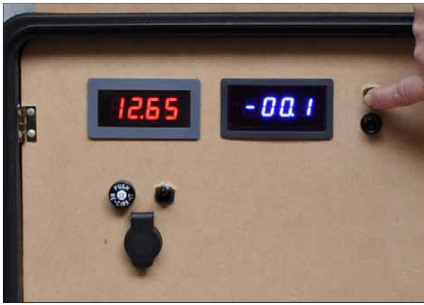
The meters only light when the button is pressed. This prevents them being left on and excessively discharging the battery. Note the merit socket, switch and circuit breaker below the voltmeter.
