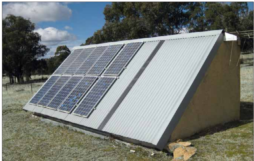
Ten 100 watt solar panels on the roof of the shed. Inside the shed are eight batteries, inverter and back up generators, plus tools, of course.
