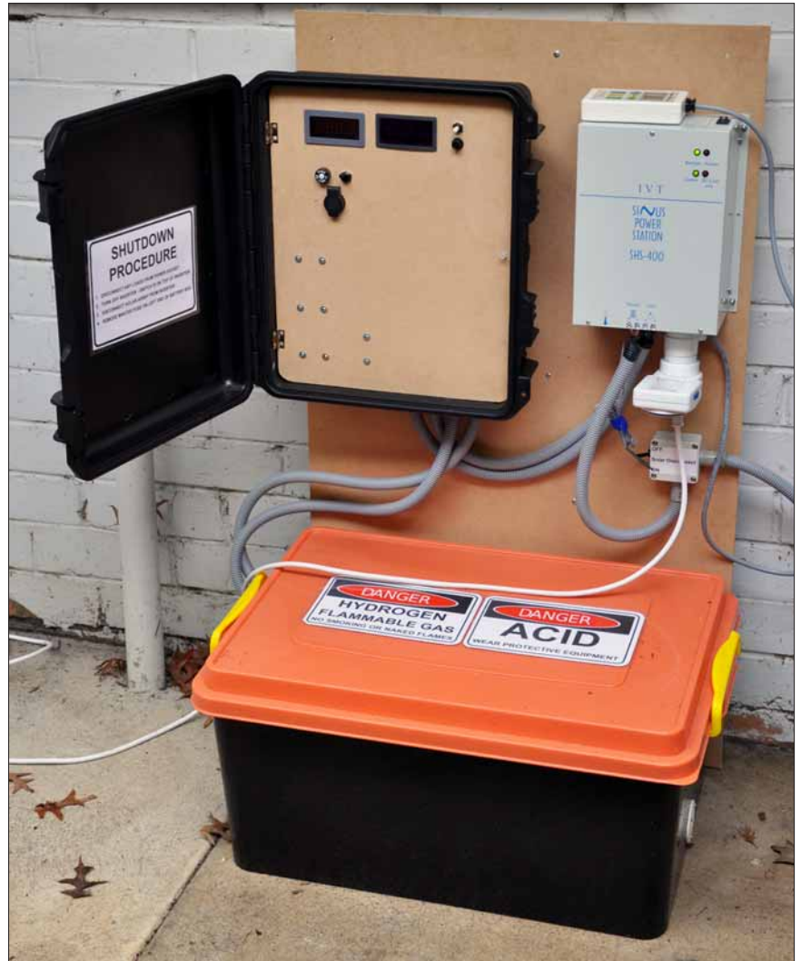
The complete power system. The bundle of wire hanging below the inverter is the solar regulator temperature sensor, waiting to be attached to the battery.
