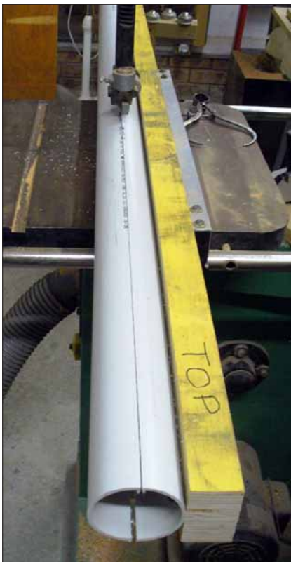
The pipes are bolted to a length of timber for easy and safe cutting.
