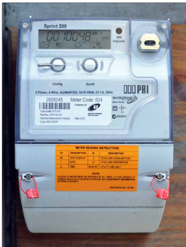
A recently installed smart meter.
