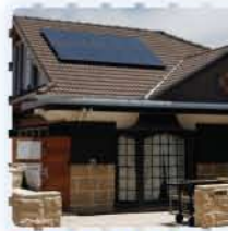
BONDI, NSW 2kw system
