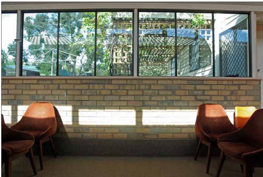
Top: Shad blades on the veranda controlling light into the home; Below: winter sun hitting the veranda wall.
