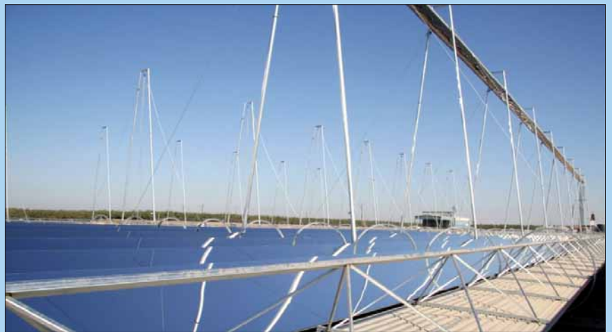
A solar thermal collector at the Kimberlina plant in California.
