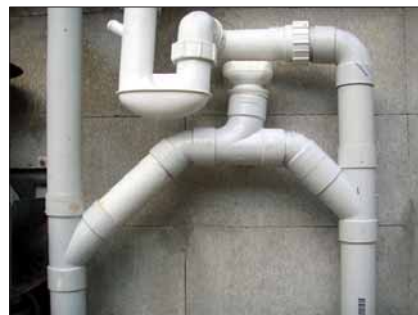
3. Overflow pipe. If the greywater can't escape fast enough, for example when the kids let the water out of the bath whilst I am having a shower, it will fill 1.5 metres of vertical pipe on the right, then overflow into the kitchen drain pipe on the left, flowing to the sewer. The air-valve is to stop airlock/siphon issues.
