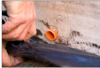
10. Cut a hole 5cm from the bottom and insert 25mm PVC pipe.
