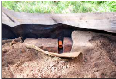
11. This drainage pipe 5cm from the bottom lets out excess water, stopping the veggies from drowning in a downpour.
