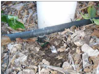
5. This is a one inch (25mm) poly and one inch poly pipe Y piece. I used the cheapest low density irrigation poly I could get. Hose clamps were not needed.
