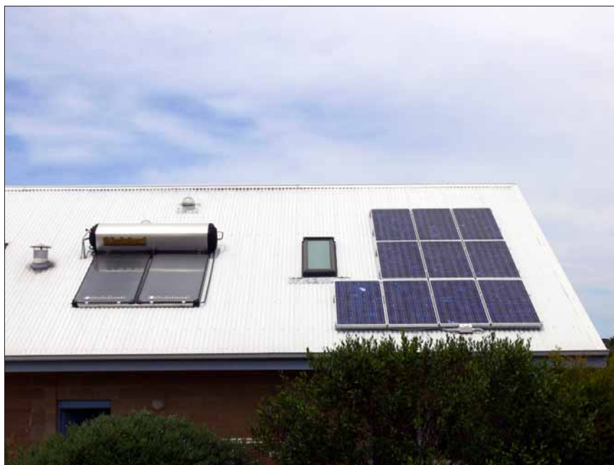
The perfect energy roof. It faces due north at an angle of 36 degrees, the same as the latitude in Malla-coota. The 'Black Chrome' Solahart was installed in 1998 and has worked perfectly. The BP Solar 1550 watt system is producing up to 10.3 kWh per day. This was Malla-coota's first grid-interactive solar system.
