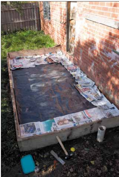
5. Place layers of newspaper over underlay to protect it from stone layer.
