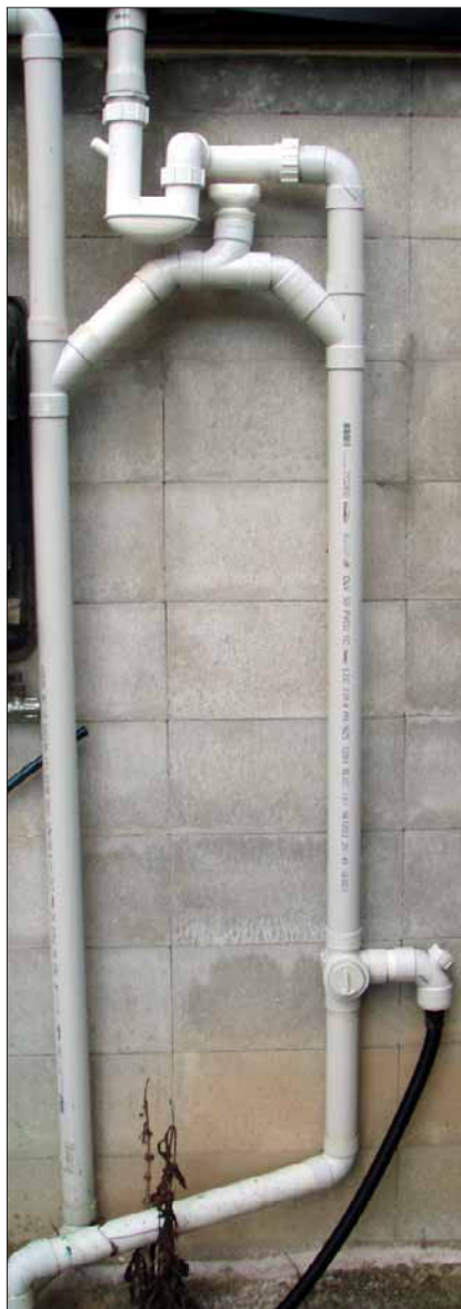
1. This odd looking contraption guarantees things work smoothly. It's an overflow pipe and diverter valve. Details on how it works can be seen at right.
