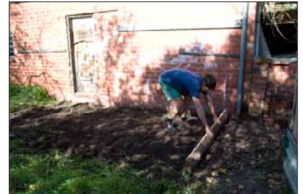
1. The site needs to be as level as possible, use a builders level to check.
