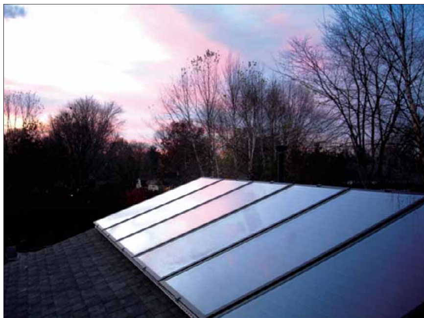
The water tank doesn't need to be on the roof with a solar hot water system. Split systems are becoming more popular.
