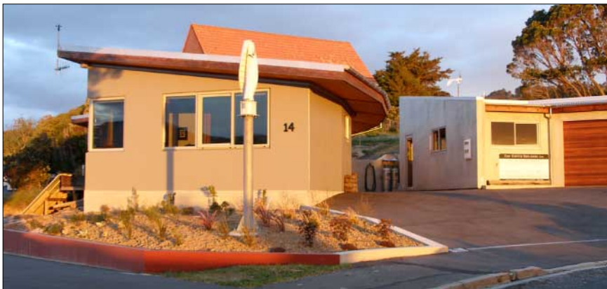
Top: The house under construction with a view over Company Bay. Bottom: The one mature native tree on the property (called a Rata, top right side of photo) flowered profusely last year for the first time, attracting two types of New Zealand native birds (the Tuis and Bellbirds). Note the two wind generators (second one on garage) and the weather station on the left side of the house roof. Harnessing the wind with the generators is a challenge, balancing visual size and noise against maximising power output. A high priority is to keep the neighbours happy on both counts. These generators are used for charging the battery bank.
