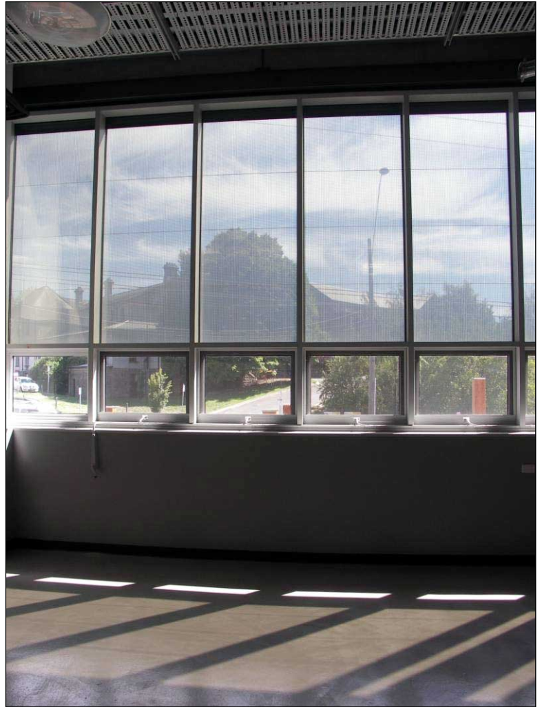
There's a view outside, despite the photovoltaic capabilities of the glass.
