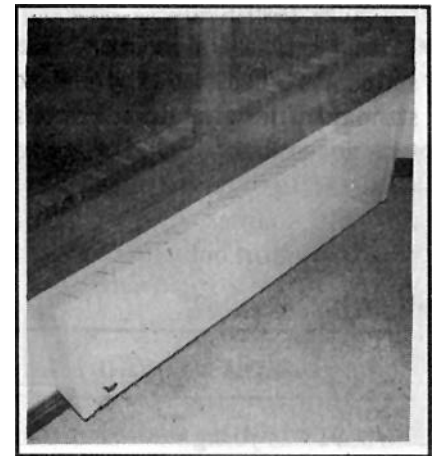
One of the heaters which is run by hot water from the "Bosky" boiler.
