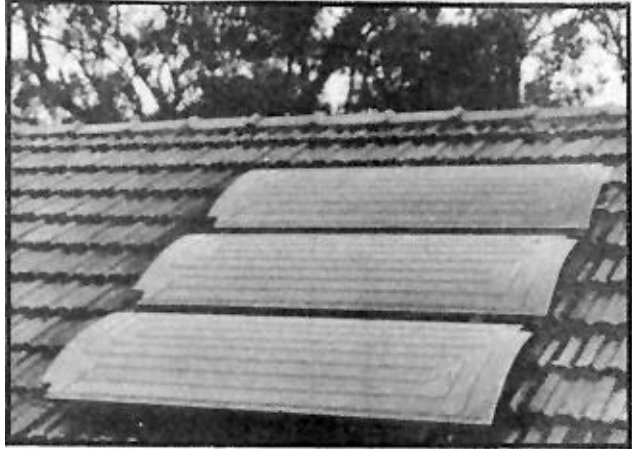
The collectors on the roof of a house.
